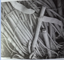
Cut and torn power and control cables
